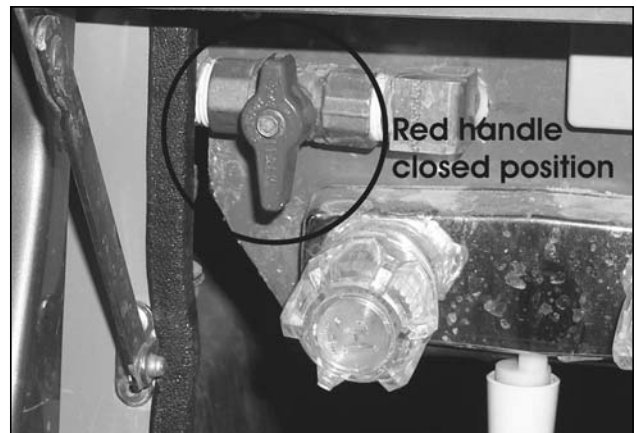
Picture G-P5: Closed position of the city water tank fill valve.
